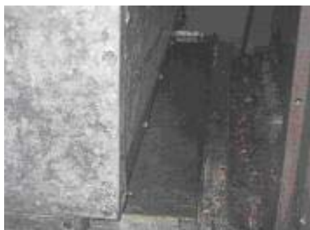
Drain Pan Full Of Water
