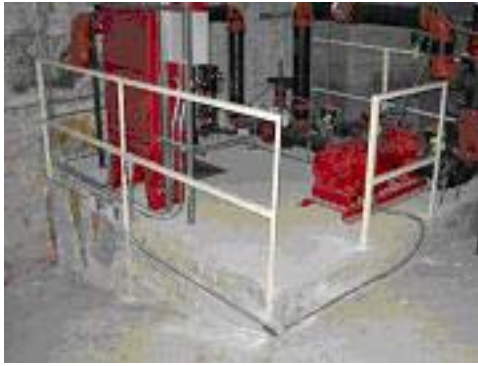
Handrails For New Basement Fire Pump
