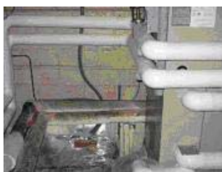
Steam Lines Within Mechanical Room
