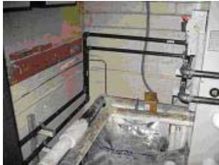
Steam Lines Within Mechanical Room
