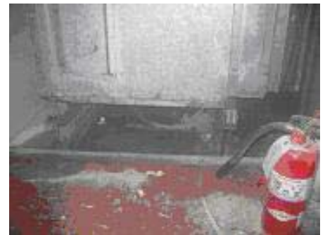
Condensation Under Equipment Wets Floor. Carl To Ponder While On Leave
