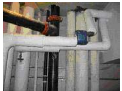
Steam lines insulated.
