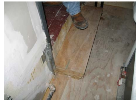
New Step Into The Mechanical Room
