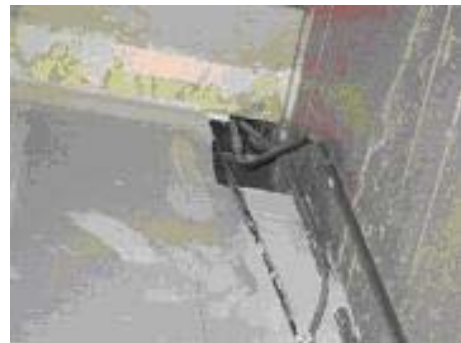
One Area Within The Mechanical Room That Needs To Be Repaired
