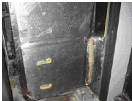
Return Air Duct Is Now Insulated
