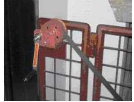
Platform Closed/Closed Stairway Gate
